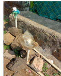
Fig. 12. Failed water pipeline
