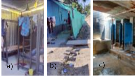
Fig.15 a), b) , c) Explaining the of worker housing in present ( source: case study visit )
