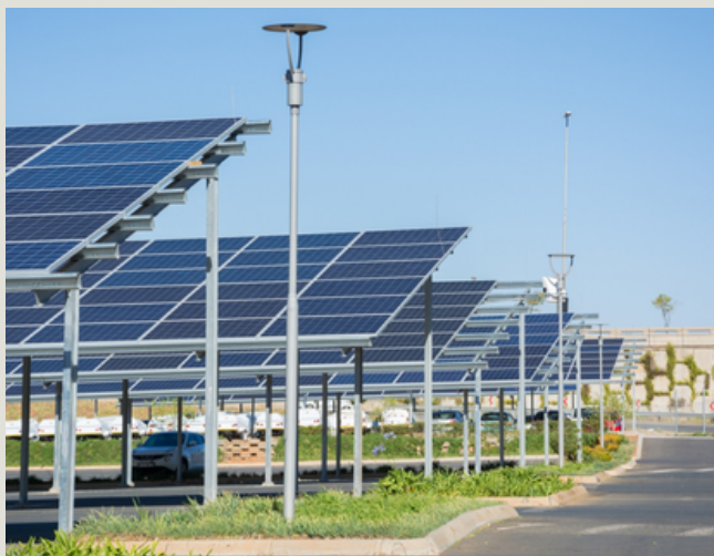
FIG 9.2.10 SOLAR PANELS ABOVE PARKING
