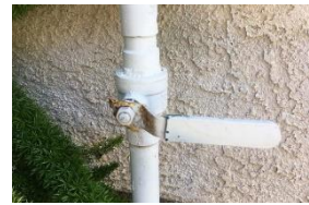
Central shut-off valve
