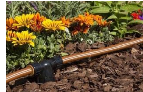
Drip irrigation system to reduce evaporation
