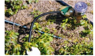
Time based controller for the valves
